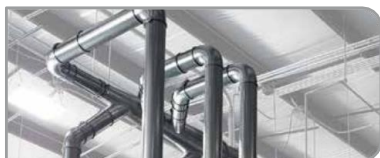
Quick-Fit Duct System installed.
